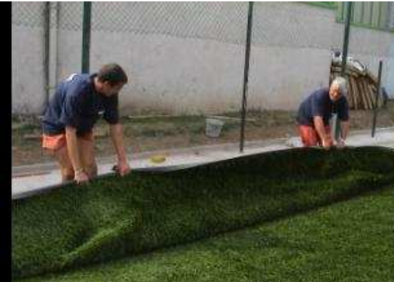
Installation of the roll of synthetic turf above the water collecting unit
